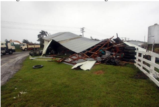
Figure 2. Light industrial building destroyed.
