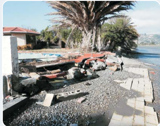
Red-zoned house facing the Avon-Heathcote Estuary – severe coastal erosion and inundation has damaged the seawall, swimming pool and house. Photo: Ian Wright, Christchurch City Council.
