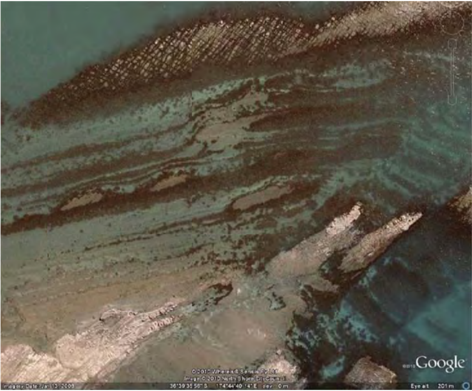
Figure 13: Google Earth aerial view from 200 m elevation showing open joint planes at Piripiti Point, Okura, north of Long Bay. This view clearly shows that the shore platform has opened along 2 sets of joint planes and is vulnerable to erosion.
